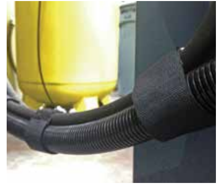
Vibratory hoses in manufacturing environments use Grip Straps to bundle expensive electrical lines.
