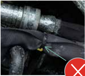
Zip tie that slipped and damaged hose sleeve.
